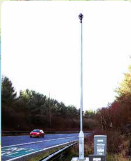
Additional CCTV Coverage
